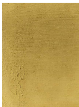
Example of Mud Cracking
