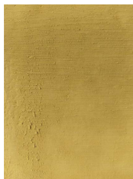
Example of Mud Cracking
