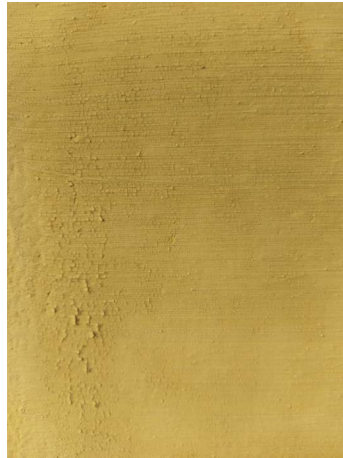
Example of 'mud cracking' when substrate hasn't been correctly 'damped down' or limewash dilution rates are not correctly observed
